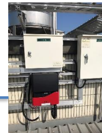
Invertor of various brands
